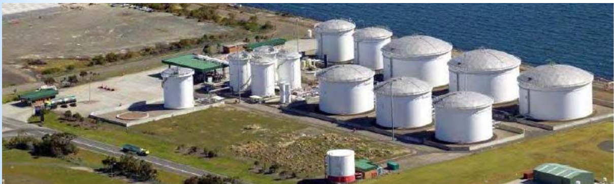
Construction has commenced on the additional 74,400 cbm of tank storage at site B
