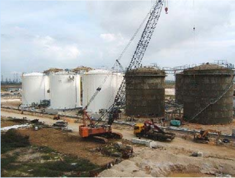
Chemical Tankfarm, December 2005
