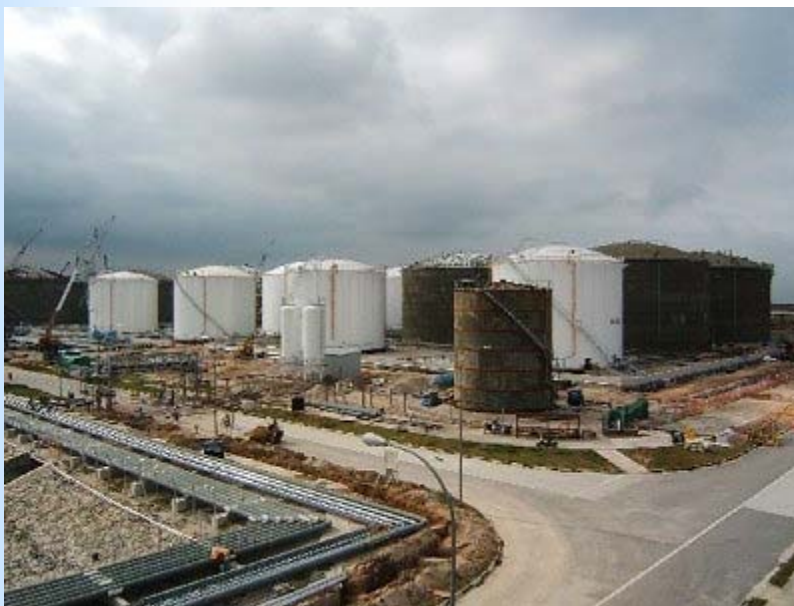
Petroleum Tankfarm, December 2005
