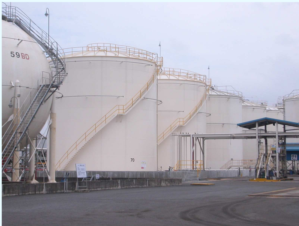
New tanks 69 and 70 in VTK Terminal 1-C
